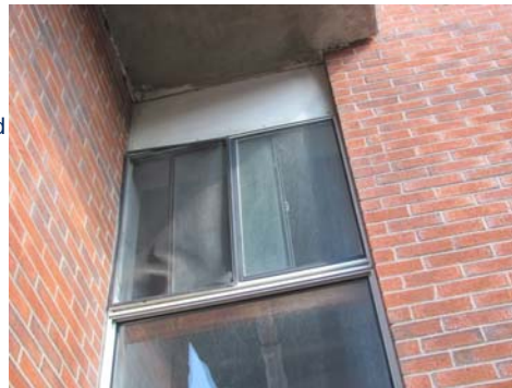
Poor Condition of Window to be Replaced
